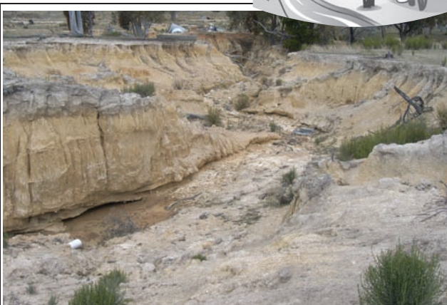
Very high to high risk: active erosion tunnels
