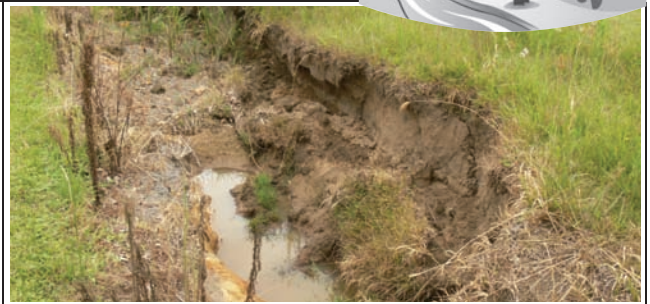
Very high to high risk: active erosion on banks <2 metres
